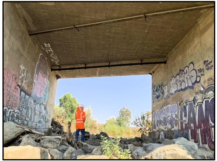
UNDERSIDE: A Caltrans worker stands underneath the Dawson Canyon Road bridge during an inspection in 2020. The bridge has hidden as well as visible pipes attached to it.
