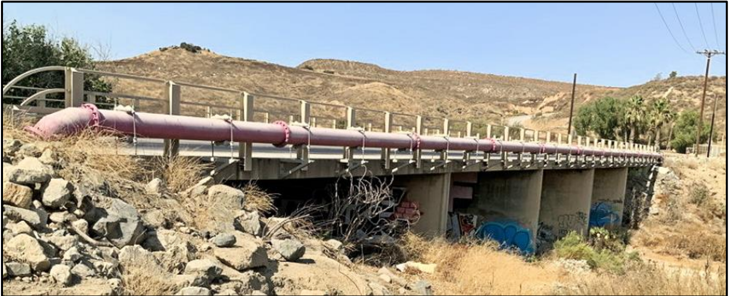
TEMESCAL WASH BRIDGE: Dawson Canyon Road and the bridge it crosses are both owned and maintained by WM and not the county. The bridge never received proper permitting by the county when WM built it. A Caltrans inspection of the bridge in September 2020 found it to be “poor and structurally deficient.” An 8-inch pipe transporting renewable natural gas is to be attached to the north side of bridge. This photo was taken during the 2020 inspection.
